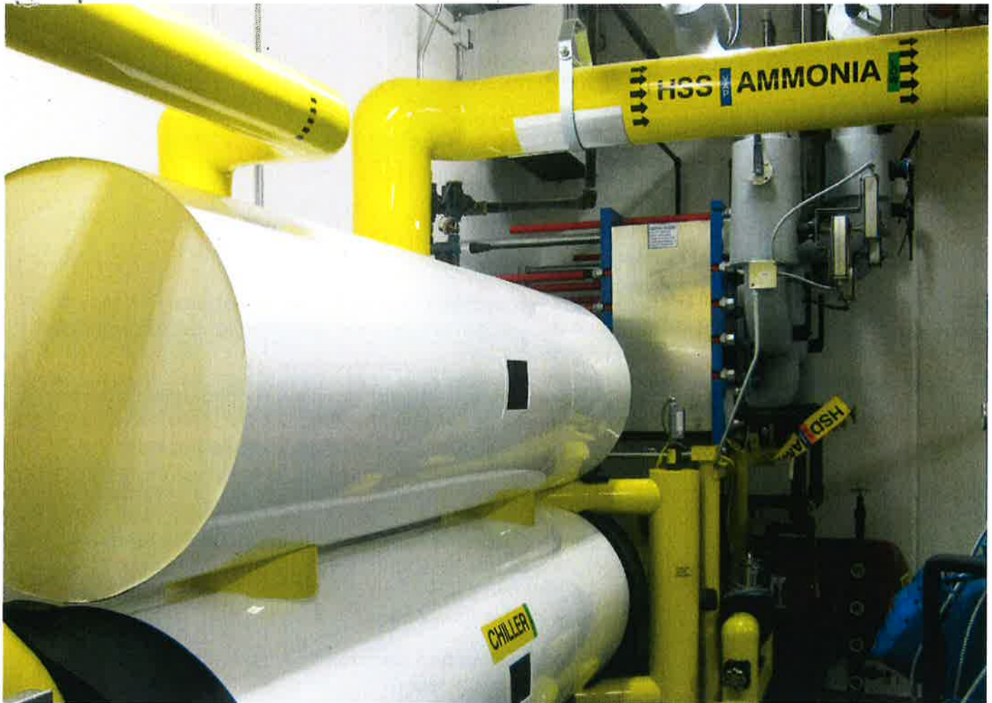
A chiller in an ammonia refrigeration system. Image Source: Stevens Engineers
